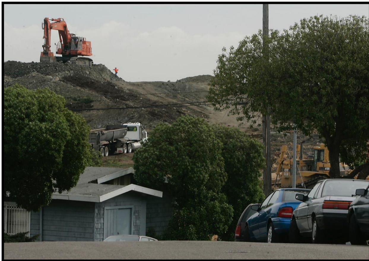
Looking through the Hunters Point neighborhood, Lennar Corp. grading the new development in 2006. 161 Source: Liz Hafalia/San Francisco Chronicle/Polaris
