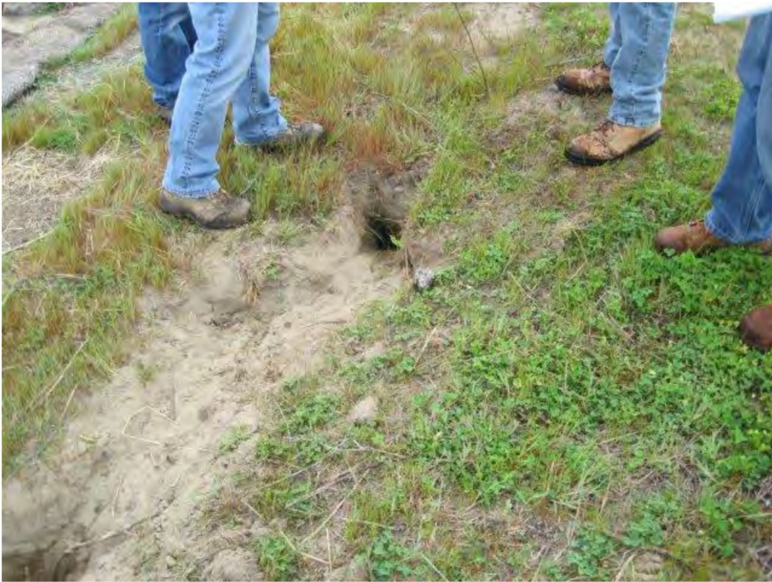
Photograph 15. Large, collapsed burrow near revetment crest in central portion. Second burrow entry at lower left corner of photograph. Burrow scheduled for repair.
